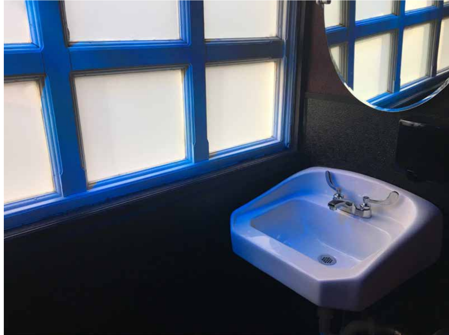
Restroom Sink, Longmont, CO, 2019
