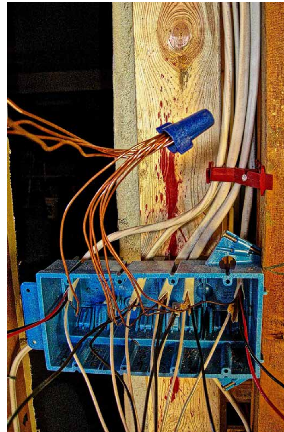
Electrical Wiring, Boulder, 2013
